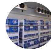
Warehouses Cold Storage
