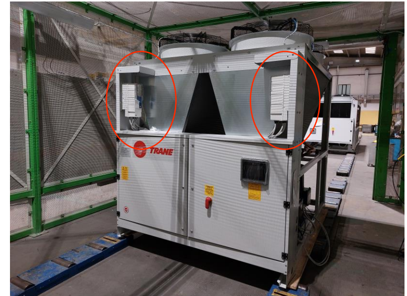
Housing of inverters device for pumps (digit 37)
